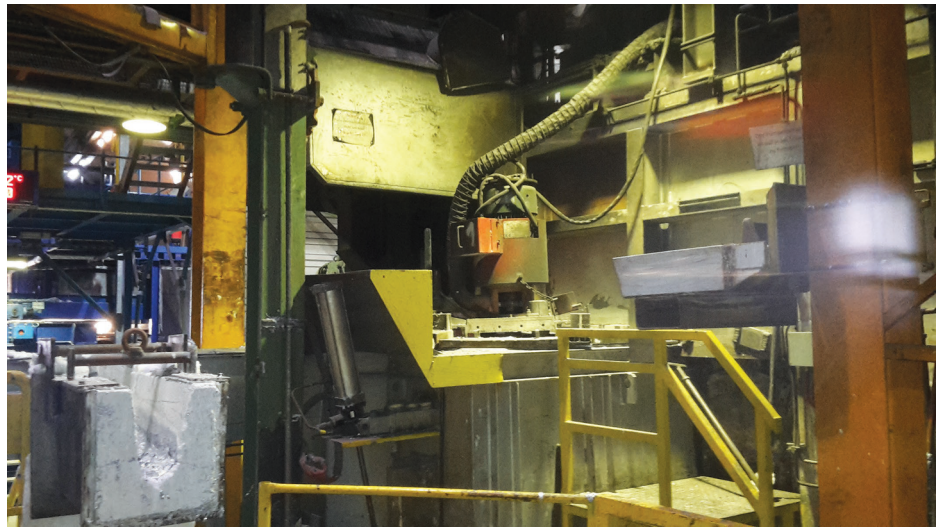
The pump in situ at Trimet.
